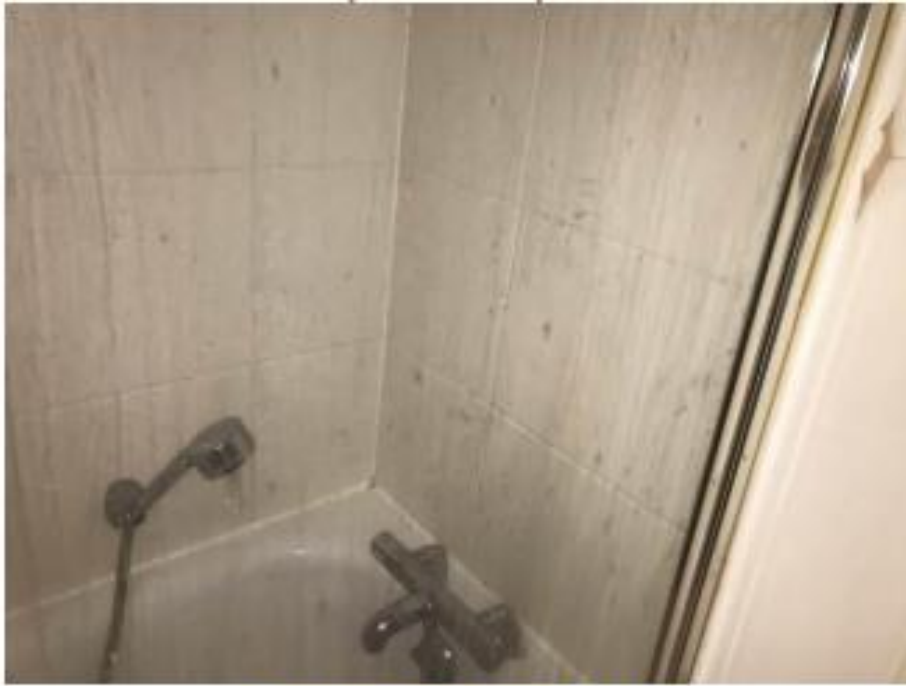
Shower screen not clean
