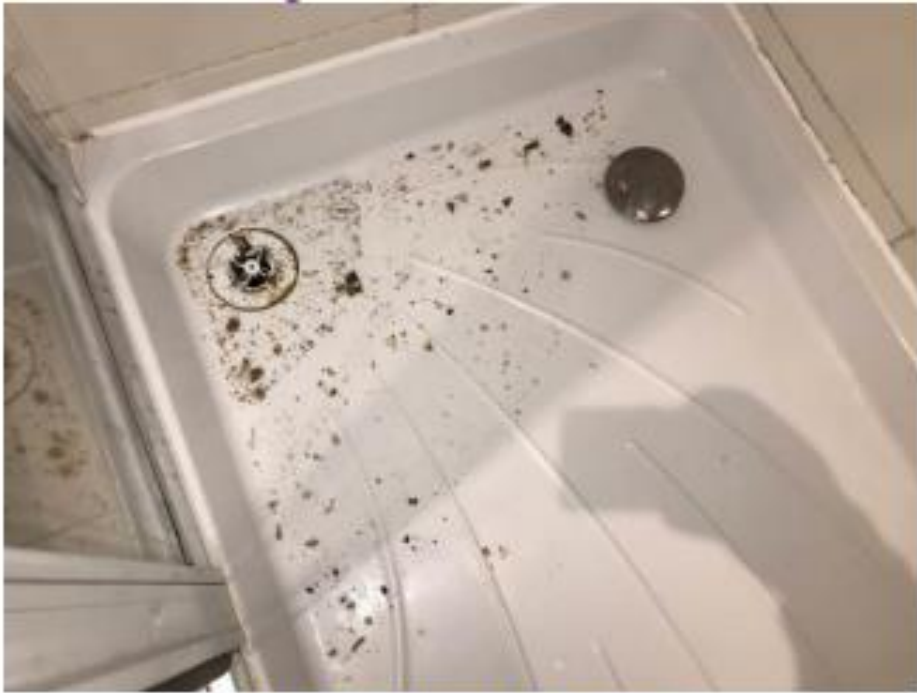
Heavy debris to shower
