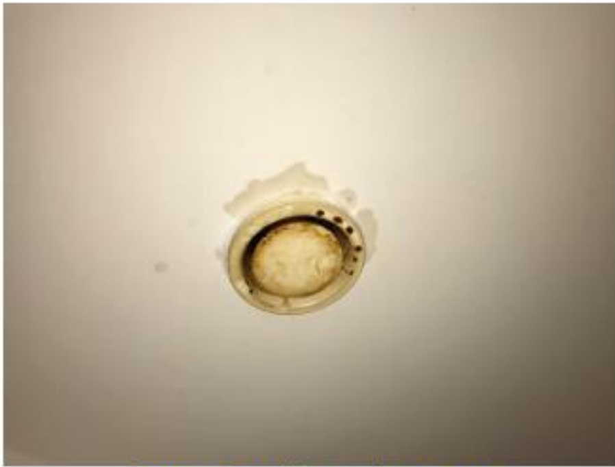
Grease to ceiling and extractor
