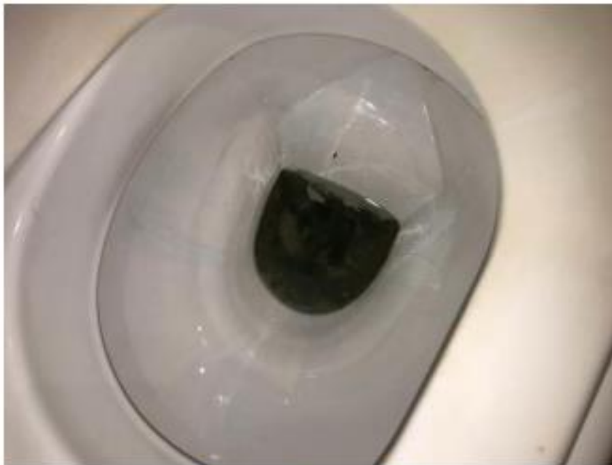
Limescale to toilet
